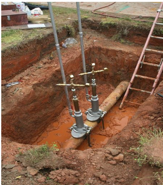
Photo of bag tubes installed, bags positioned and inflated, courtesy of David Payne, PLCS, LLC.
