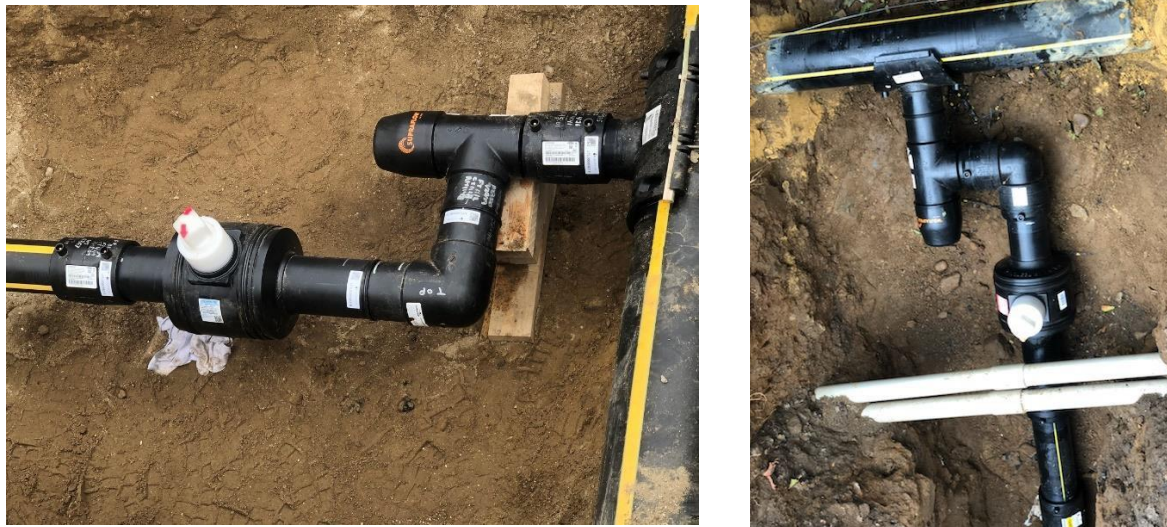
Photos of “Supraflow” Tee branch connections as used in the field, courtesy of David Payne, PLCS, LLC.
